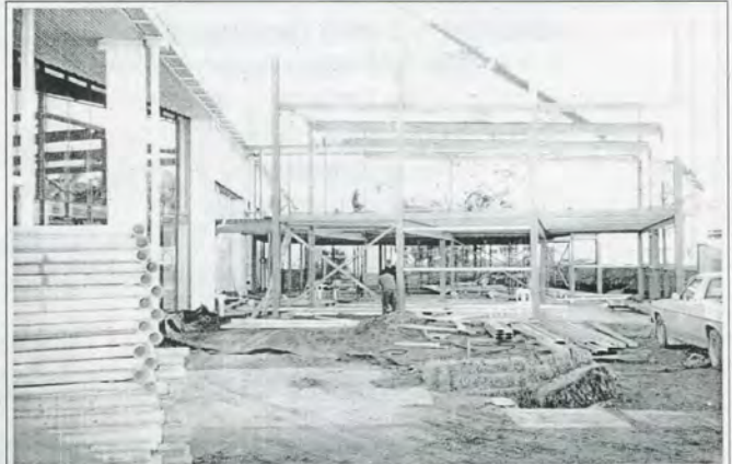
Stage 4 Museum extension under way. This framework is now completely covered and the first floor deck is completed and extends over the shop area to the level of the Function Centre. The fill removed from the site is being used at the airfield side of the Museum for viewing mounds. Peregrine
